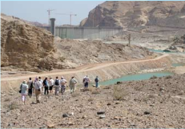
The Wadi Daiqa dam in preparation and in the foreground shallow marine sandstones of the Amdeh 4
