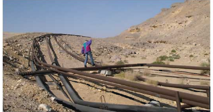
Flow lines cover Jebel Fahud, taking oil from the wells to centralised facilities
